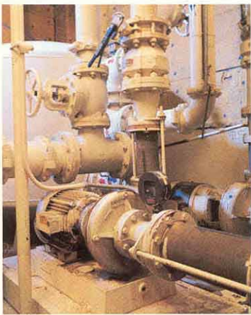
The egret fountain is operated by a 300-gallon-per-minute pump (above) that circulates water from the reflecting pool.
